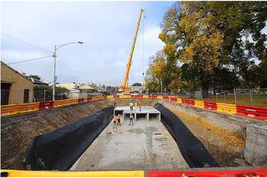
Melbourne City Council is installing a stormwater tank under Darling Street, East Melbourne which is expected to save 20 million litres of water a year. Photo: Craig Abraham
